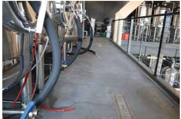
Elevated Brewing Area
